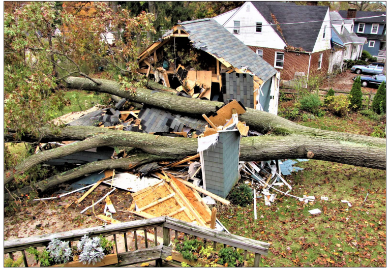
The heartbreaking loss of the two Pontiacs after the oak tree uprooted and fell on the garage.
